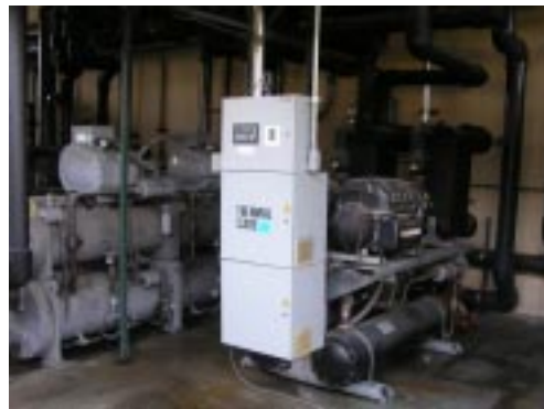
Thermal Care TCW140HE central chillers with dual, frictionless, oil-free compressors.
